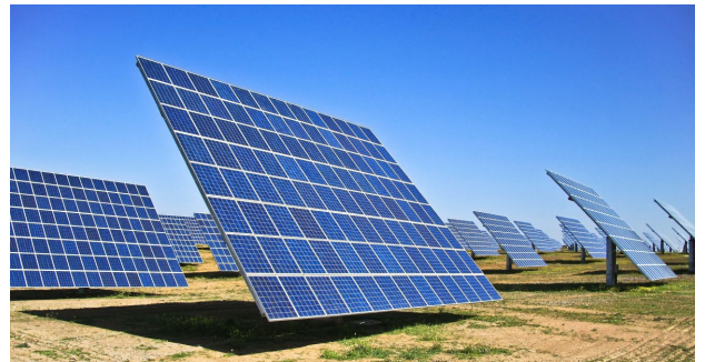
Centrale solaire photovoltaïque d'Amareleja – Portugal Photographe : Vitor Oliveira (CC BY-SA 2.0 DEED)
